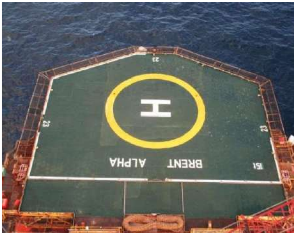
Helideck refurbishment using Humidur® FP with minimal surface preparation in offshore UK, North Sea
